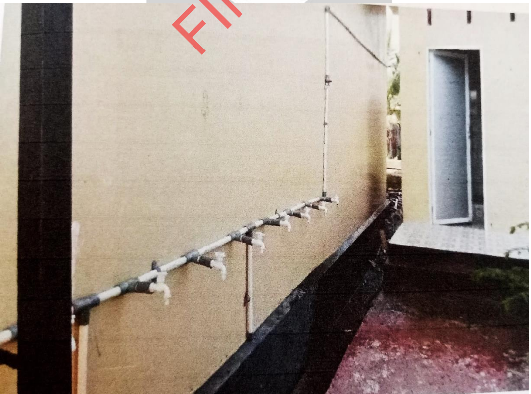
Kran wudhi/cuci tangan
